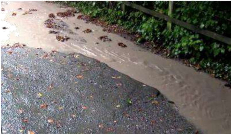
Surface run off after rain.
