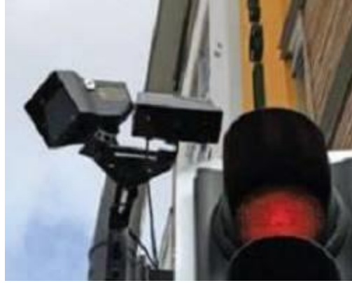
Pedestrian crossing sensor
