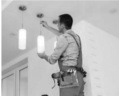
Installed light fixture
