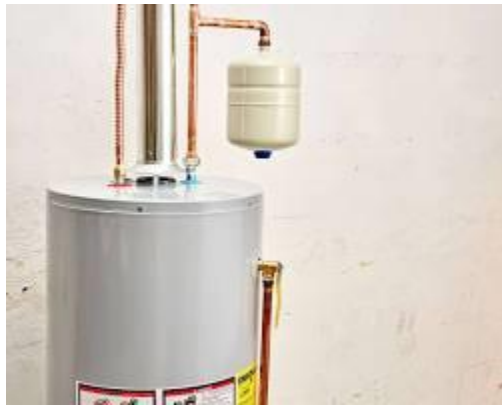
installed water heater
