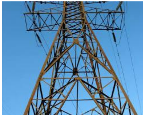
high voltage transmission towers
