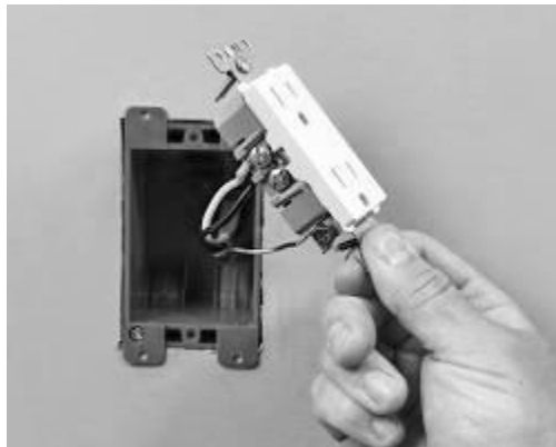
Installed wall socket
