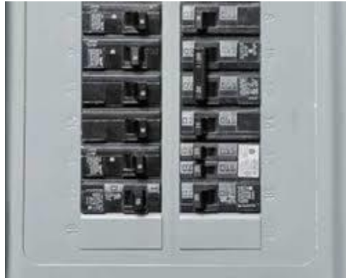
Circuit breaker panel
